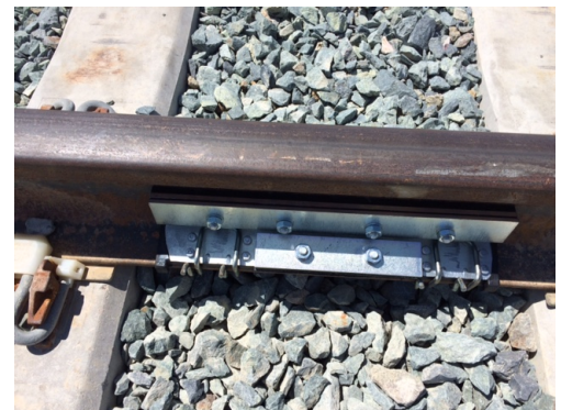
Tuned Dampers on ballasted track
